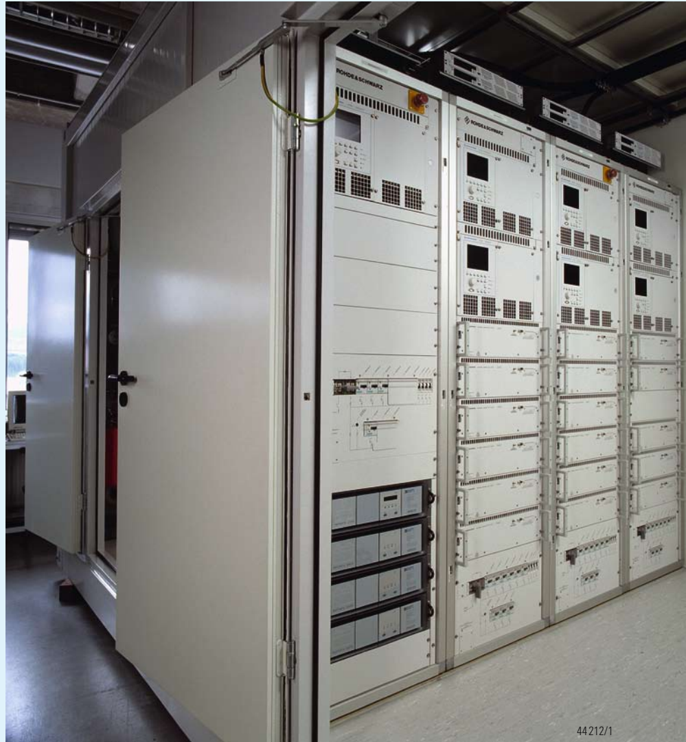
Setup of a turnkey lightweight cabinet with DVB-T transmitters of the R&S® NV/NW 7000 family for the Braunschweig site. Two transmitters each with exciter standby are accommodated in one rack to ensure optimum usage of space. In the cabinet, three racks were fitted with two transmitters each and one rack with one transmitter. Three separate cooling circuits supply the transmitters.
